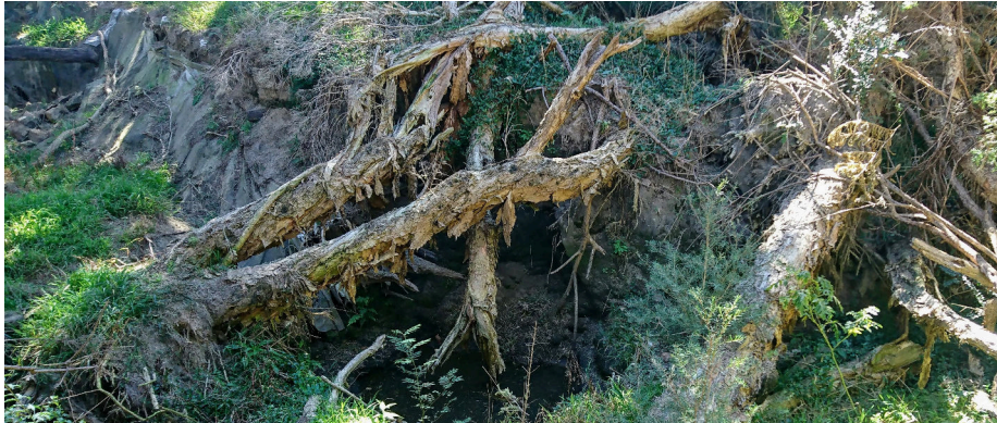
Figure 4.5: Sinkhole in Main Swamp. Note the vertical banks and the mature Melaleuca that have collapsed into the hole. Stabilising works can be seen along the some of the bank.
